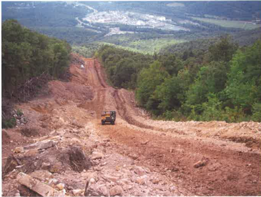
Figure 4. Example of construction road with adjacent pipeline trench. Material excavated for the road is piled on uphill side of road; material excavated for the trench is piled in a berm on downhill side of trench.
